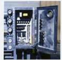
Class I, Division II Control Panel
